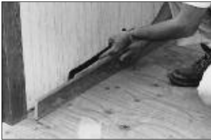
Carefully remove all existing wall base, trim, and transition moldings using a pry bar.
